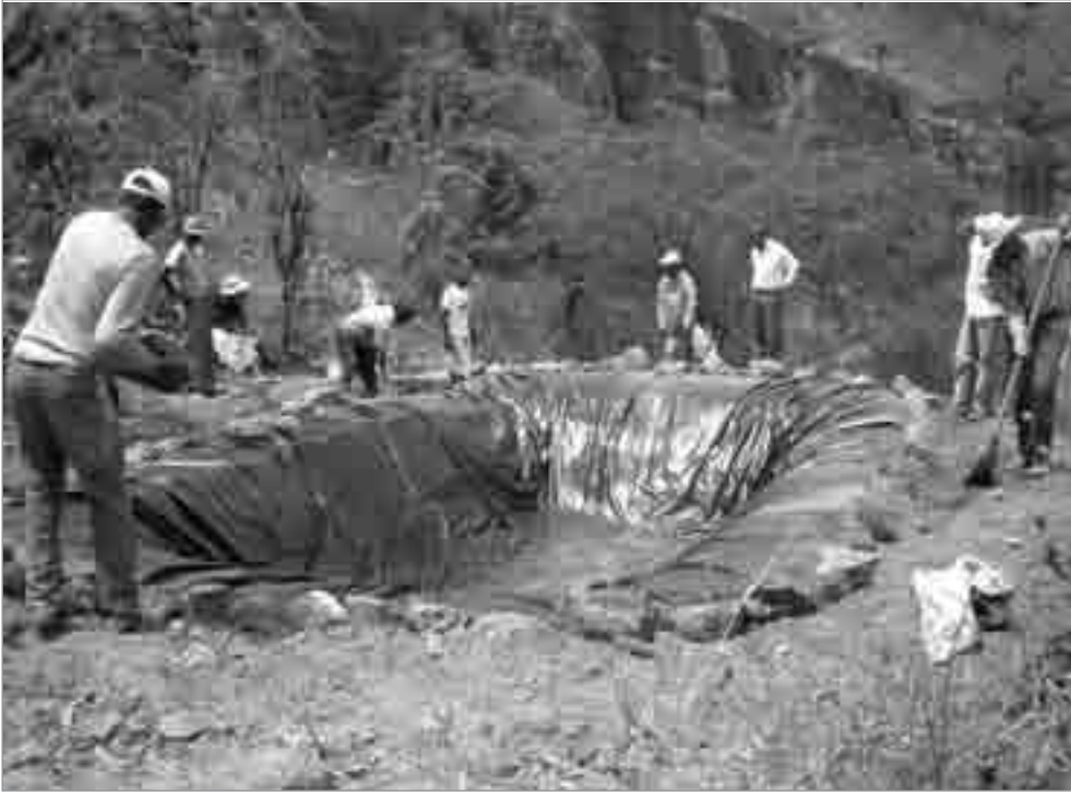
Figure 7: A minga or work party helps a colleague install his first geomembrane tank.
